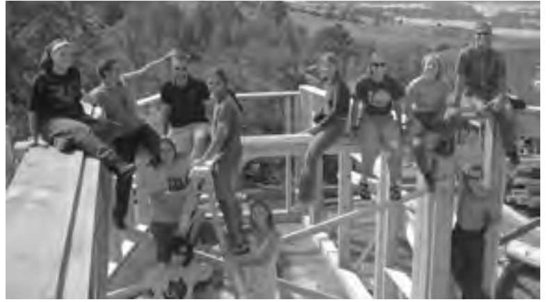
The August 2003 SCI camp and refuge staff worked hard to get Gene's Kitchen built. Thanks to Kathy, Ricardo, Simon, Annie, Pablo, Marco, Patricia, Inge, Abby, Ginny, Harry and Nelson for all of your effort. Photo by Kent Weber
