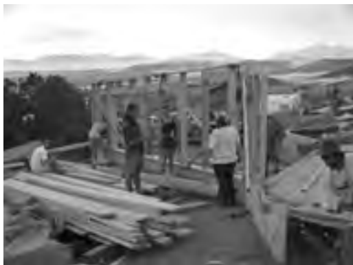
Construction has hit full swing on Gene's Kitchen. Photo by Annie White
